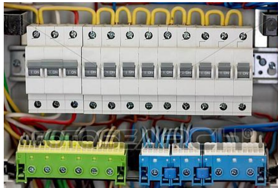
Electrical Fuse Board
