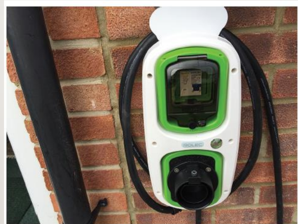
Figure 7.4 Domestic charging point
