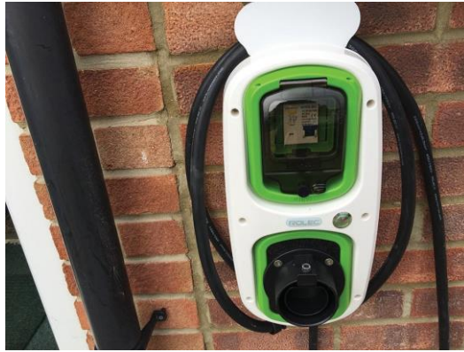
Figure 6.4 Domestic charging point
