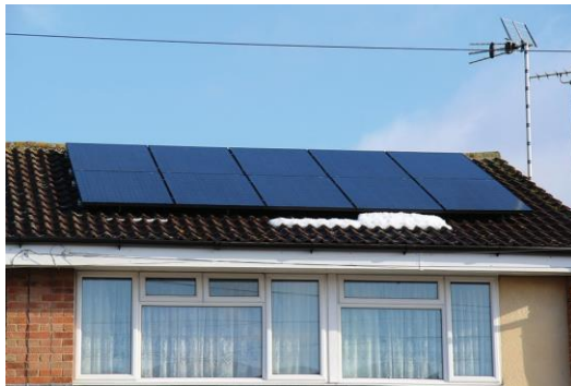
Figure 6.26 A 4kW array of PV panels (ten front and six more at the back)
