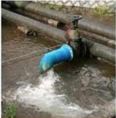
Secondary water supply
